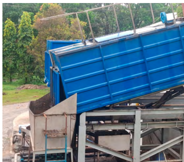
Our dewatering container being tilted to send the POME sludge to the aerobic compost therefore preventing most of the potentially methane generating solids from reaching the ponds
